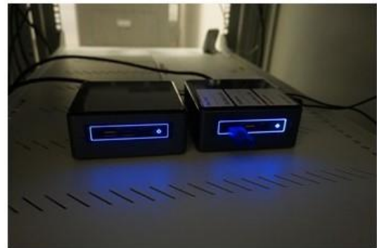
Figure 27: Validation of the Environmental Monitoring Solution regarding technical equipment
